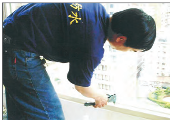
步驟四:灌注孔拉釘補孔 step four: injection hole nail fill the hole
