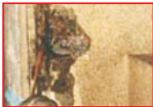
劣化處打鑿清除表面粉塵 Chisel inferior places, clean dust on surface
