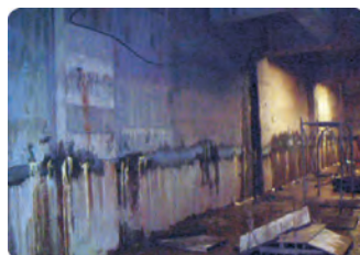
二次接縫止漏 Second joints leaking sealing
