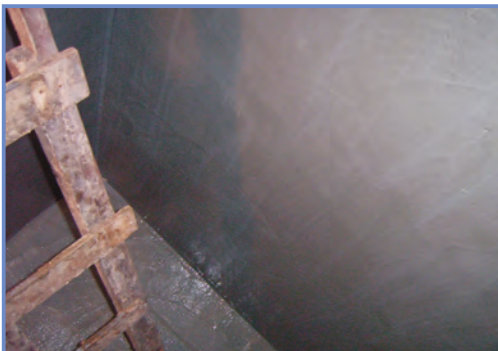
蓄水池防水 water Tank waterproof
