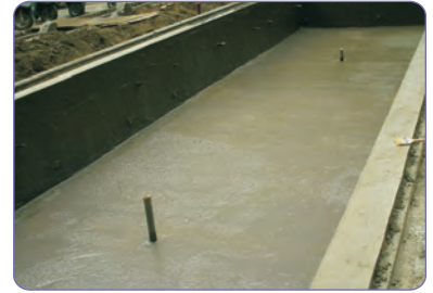
蓄水箱 Water storage tank
